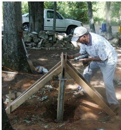
Encased between sheets of plywood and braced by 2x4s, the tombstone cures for several days before soil is packed around the base.
