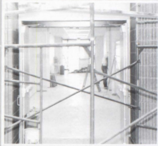
Standing tall A workman's scaffold frames the entrance to the new commons area of the high school.
