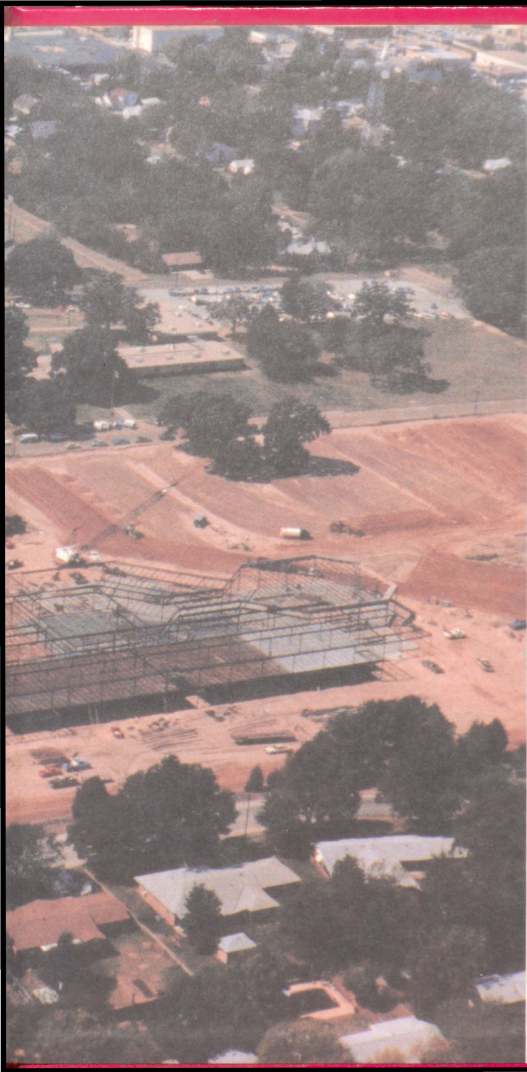
An aerial view of the new high school taken in October of 1985 shows the early stages of construction.
